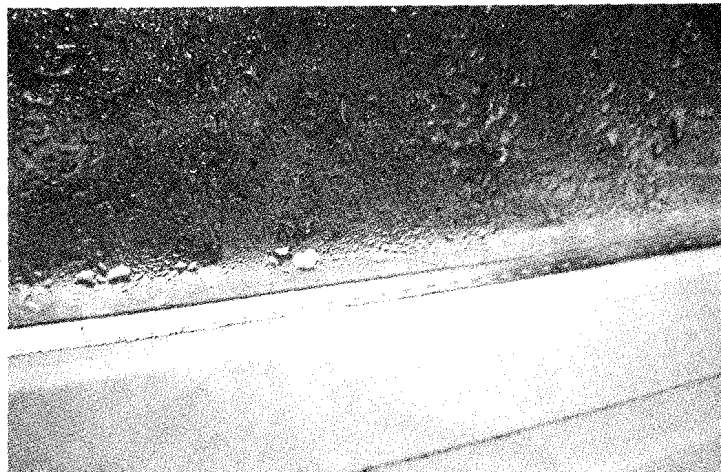
Tightly sealed windows can cause excessive condensation.
